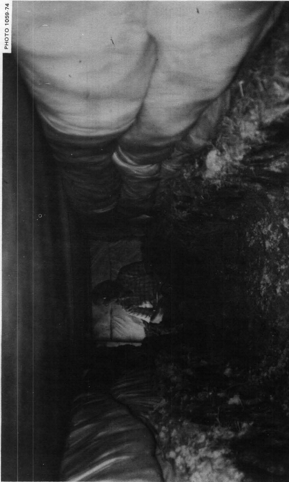
Fig. 5.12. Interior of the shelter, showing the roofing doors sloping from the right to the left, and bowed downward about 1 in. due to the 15 in. of wet earth covering them. This bowing occurred as soon as the doors were covered and did not increase during the following days.
